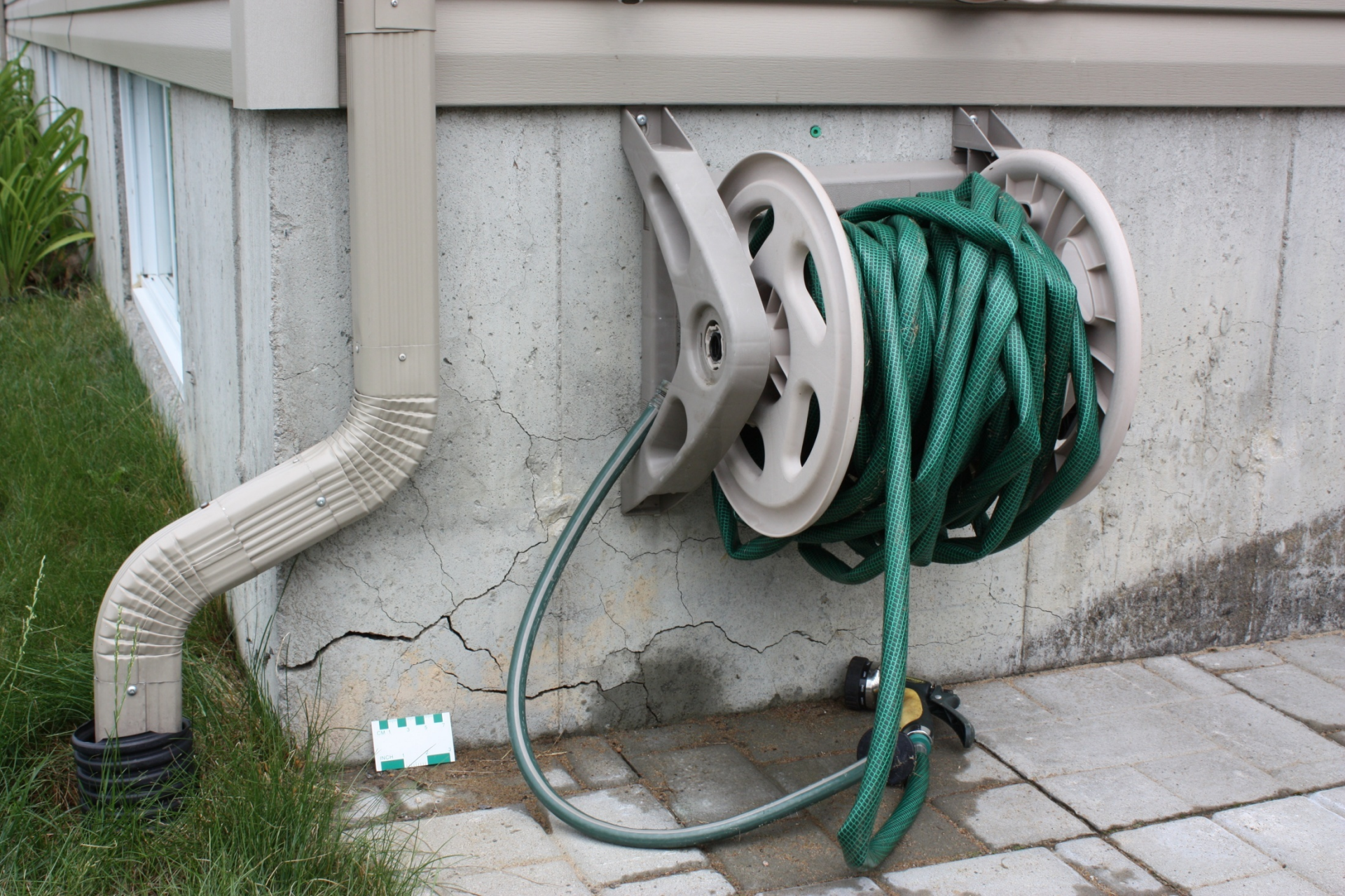
Trois-Rivières showing signs of deterioration
